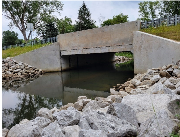
Figure 16: An example of a pre-cast concrete box bridge. (Miller Road Bridge, over Honey Creek (STR 10981), Scio Township)
